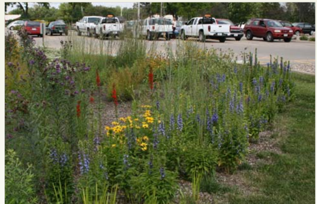
A rain garden project near the parking lot at Johnston City Hall. The rain garden was designed and installed by Community Development staff .
